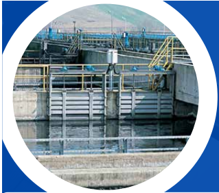
Flow Control Equipments
